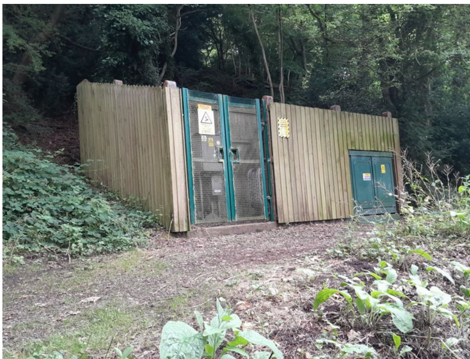
Electric substation on MHT land by Holywell Road
