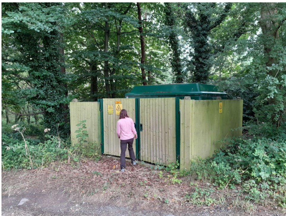
Electric substation on MHT land at Malvern Common.
